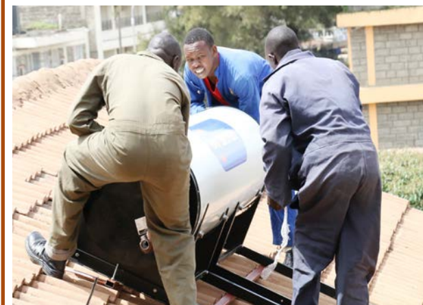
Orb Energy technicians installing solar water heating panels at Abbey Resort, Nakuru.
